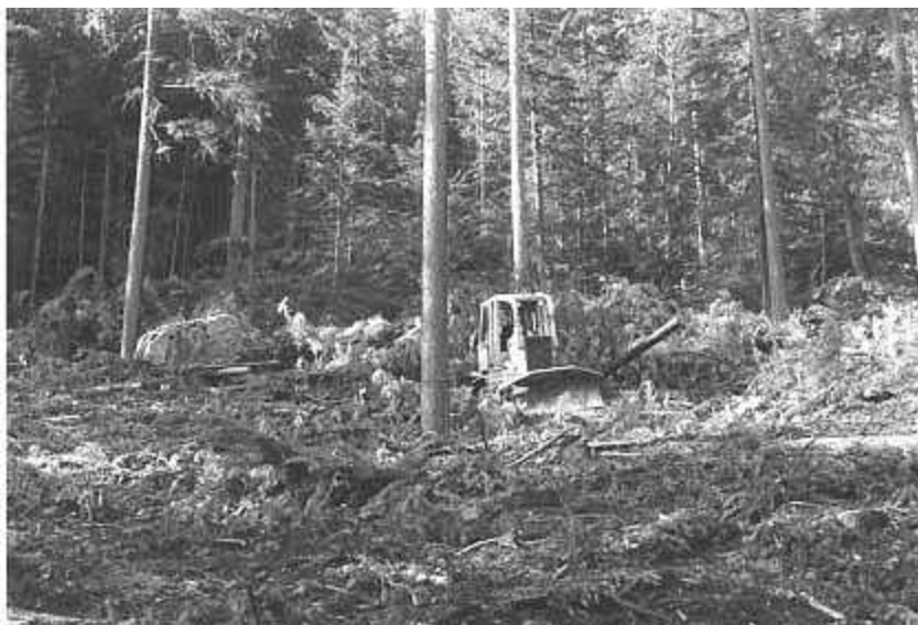
Figure 1. In Block 5, the crawler-tractor worked around reserve trees that had been marked prior to harvesting.
