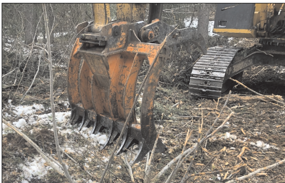
Figure 3. Image of excavator with modified brush-rake attachment used to collect fine fuels in the Burns Lake Community Forest in mechanically raked fuel treated units.
